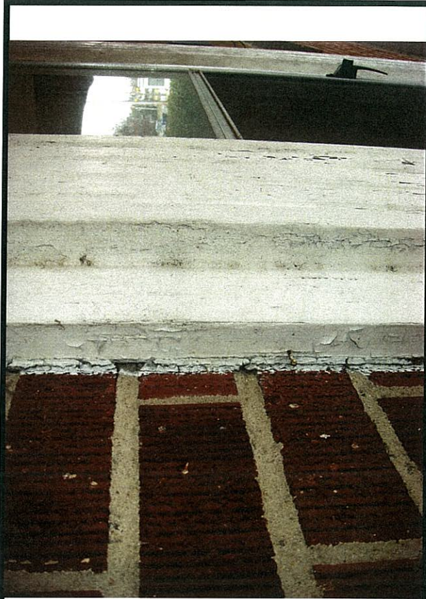
Asbestos Containing Door Caulking on Exterior doors
