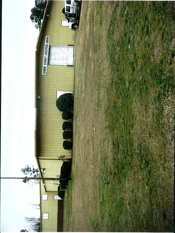
Livestock Arena . Assumed Asbestos Containing Roofing mastic and Sealants
