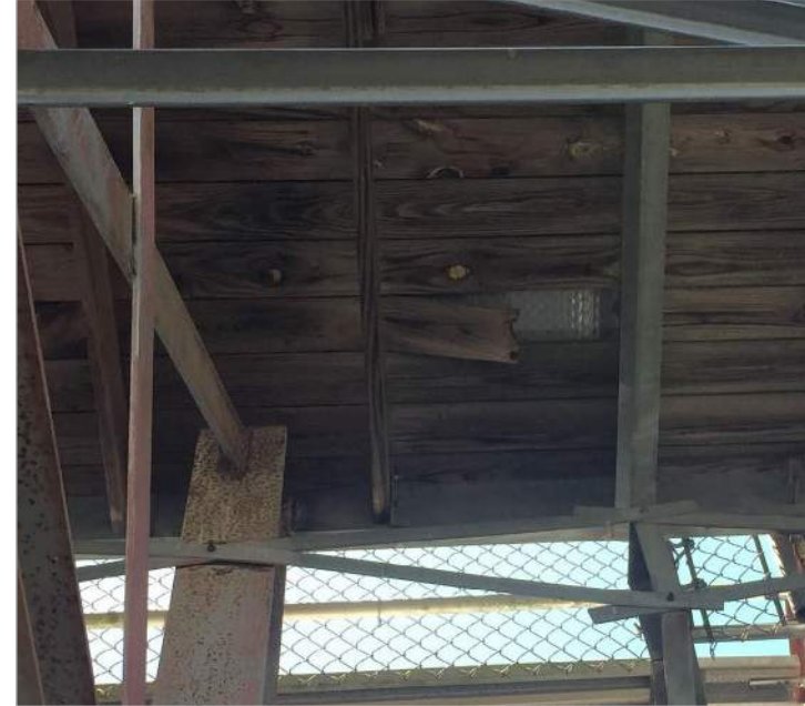
Photo 3: Damaged deck board covered by steel checker plate.
