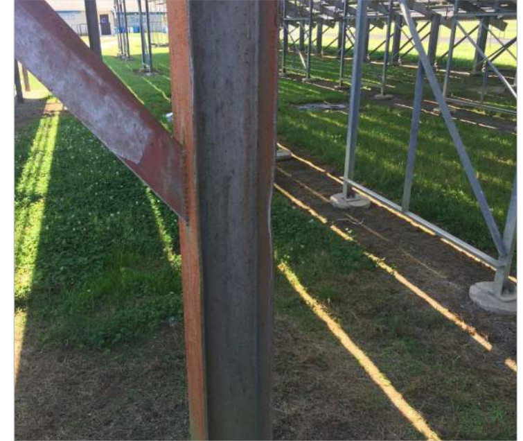
Photo 4: Damaged flange of press box support column.
