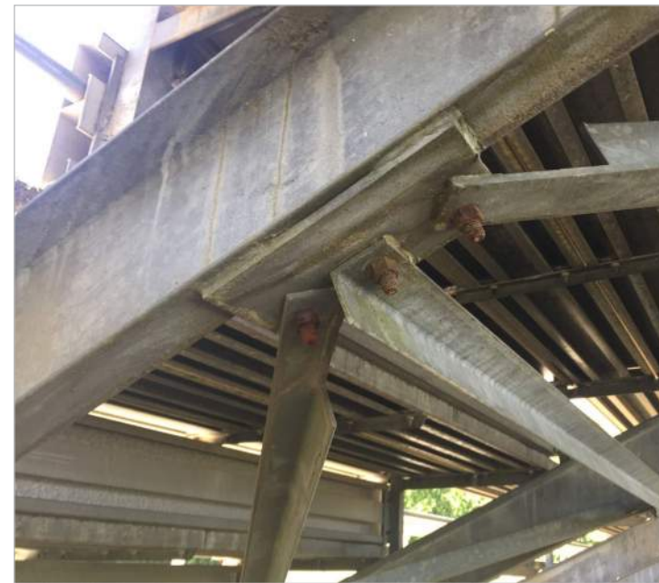
Photo 5: Representative surface rust on bolts.
