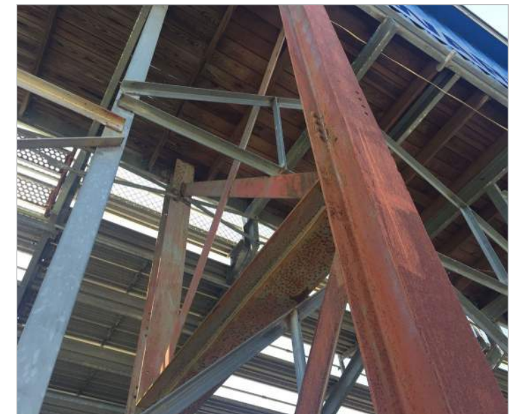
Photo 2: Surface rust on press box supporting steel.
