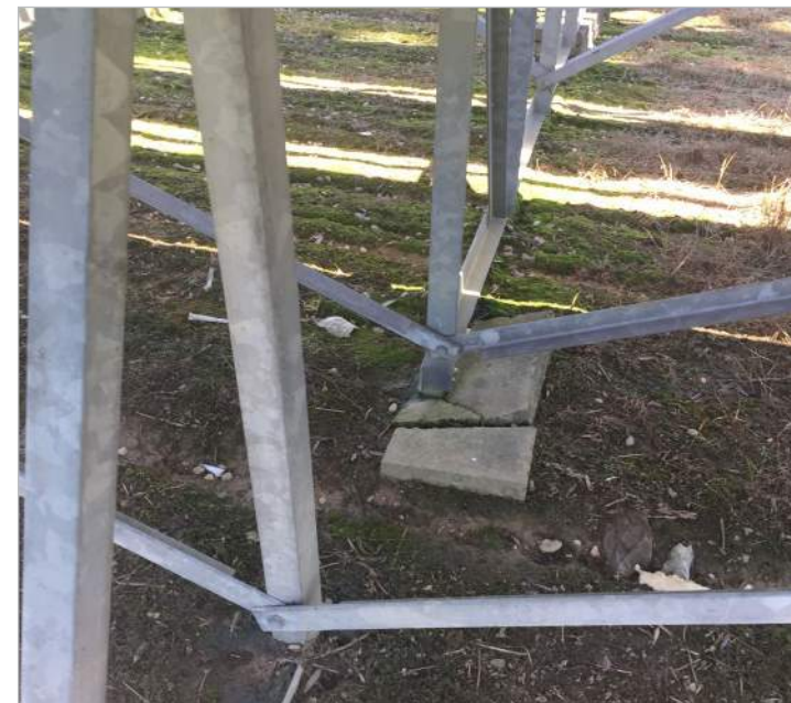
Photo 9: Cracked concrete block support.
