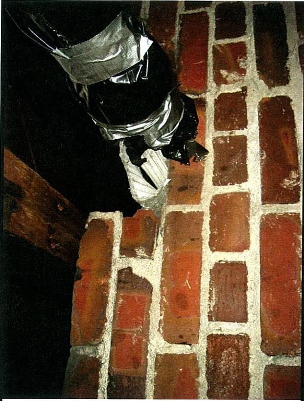
Asbestos containing Aircell pipe insulation on 2inch boiler lines throughout basement and crawl space
