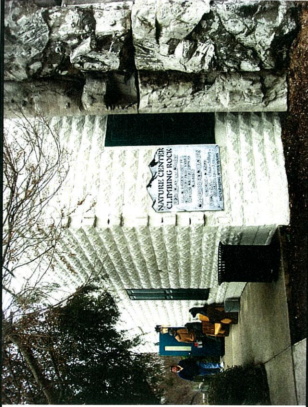
Nature Center Building with assumed Asbestos Containing Built up tar roofing and Assumed Asbestos containing Vibration Dampers
