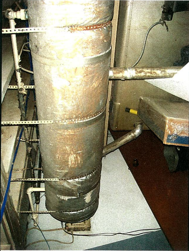
Asbestos Containing insulation on Expansion Tank in Basement
