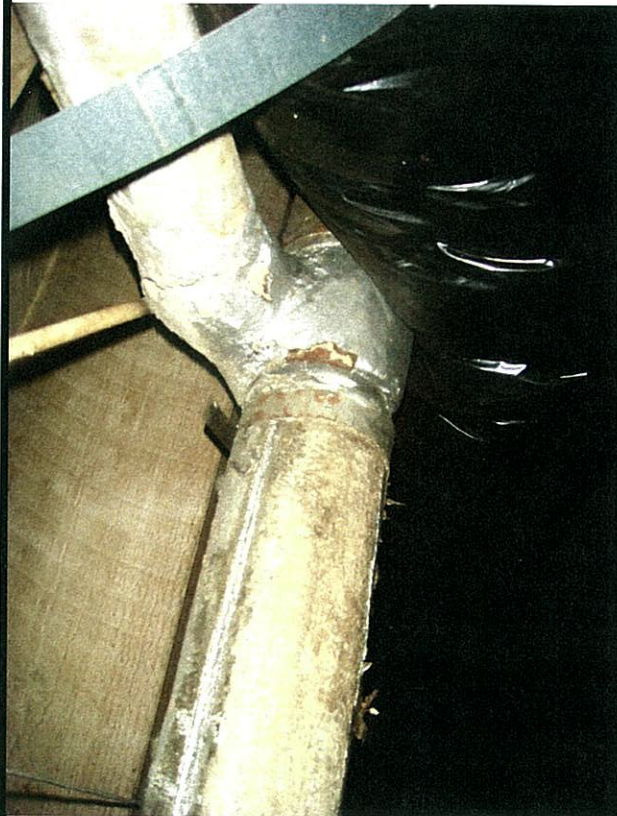
Asbestos Containing Hard elbows on hot water lines in the crawl space and basement
