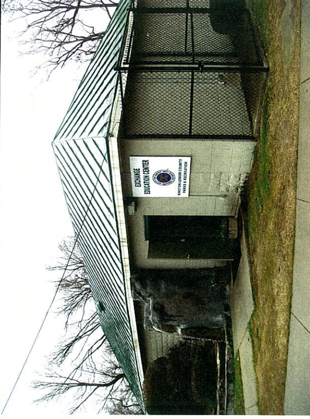
Education Building with Assumed Asbestos Containing Paint coating on metal seamed roof
