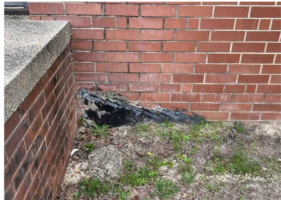
Photo #10 Asbestos-containing waterproofing mastic (HA #11)
