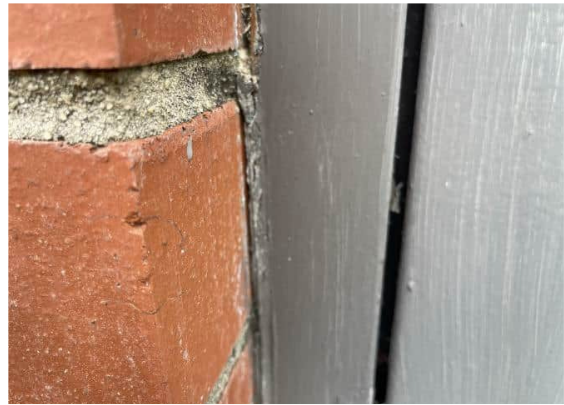
Photo #8 Asbestos-containing gray door caulk (HA #8)
