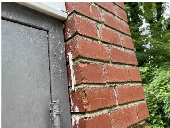
Photo #27 Non-asbestos white door caulk residue (HA #29)
