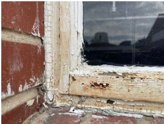
Photo #25 Asbestos-containing white window caulk (HA #26) and non-asbestos white window glazing (HA #27)
