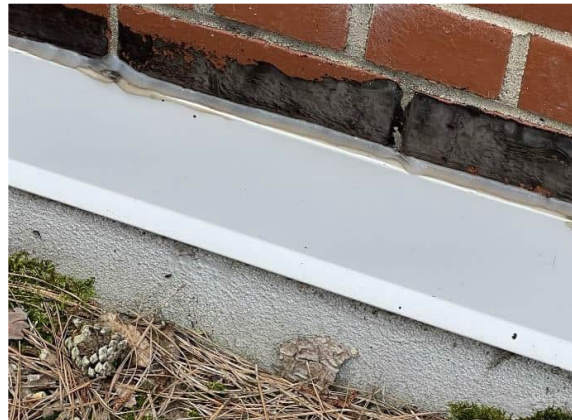
Photo #16 Non-asbestos black wall mastic (HA #16) and non-asbestos silver paint/roof flashing (HA #17)
