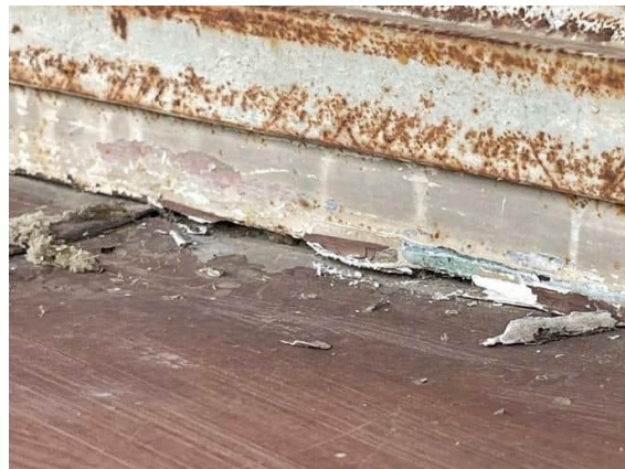
Photo #6 Asbestos-containing white window caulk (HA #6)
