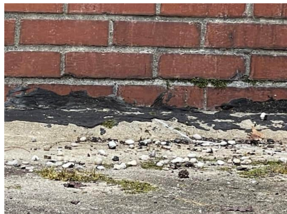
Photo #28 Asbestos-containing black wall mastic (HA #30)
