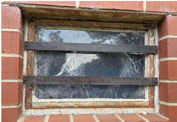
Photo #9 Asbestos-containing white window glazing (HA #9) and asbestos-containing gray window caulk (HA #10)
