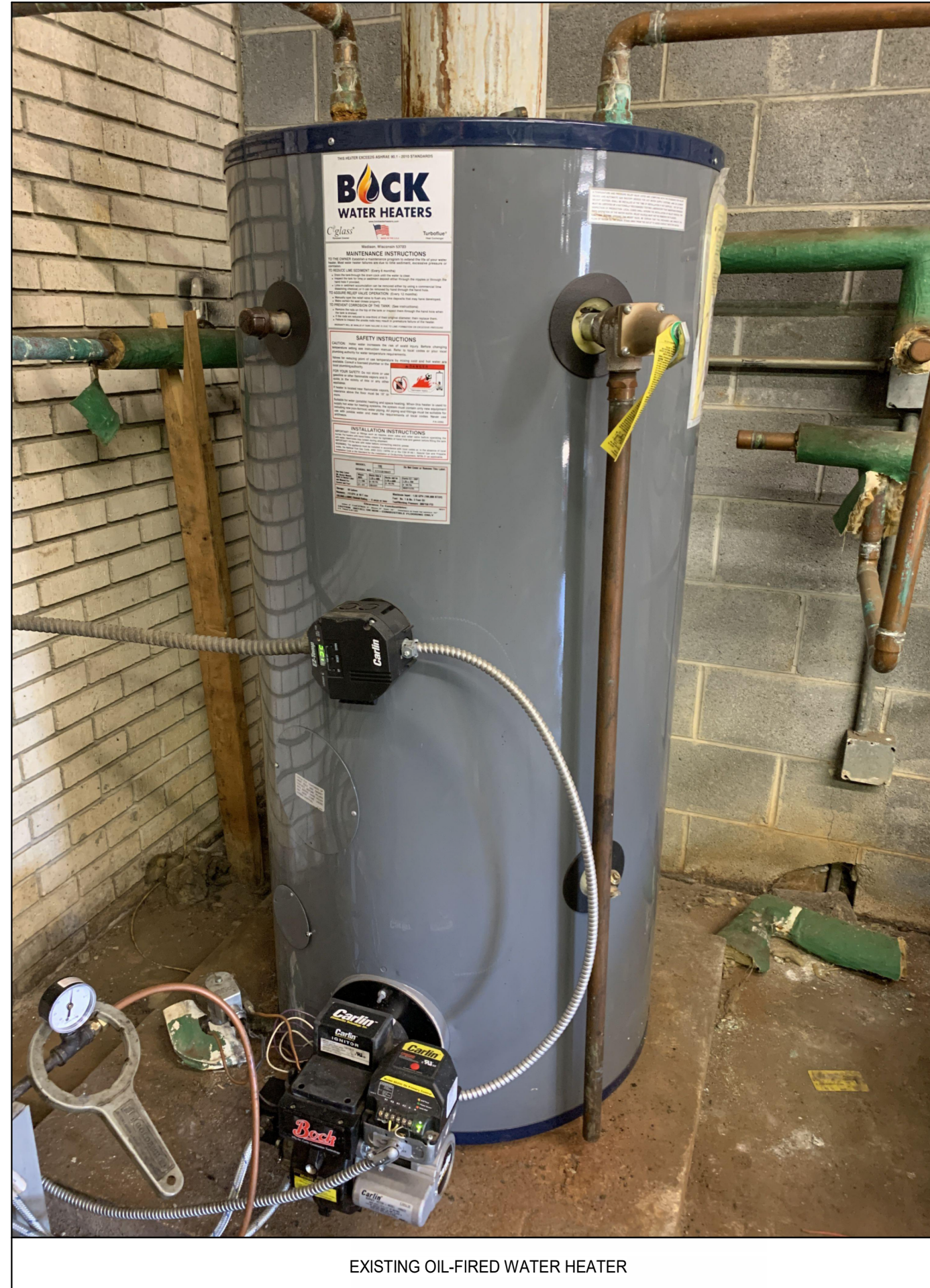
EXISTING OIL-FIRED WATER HEATER
