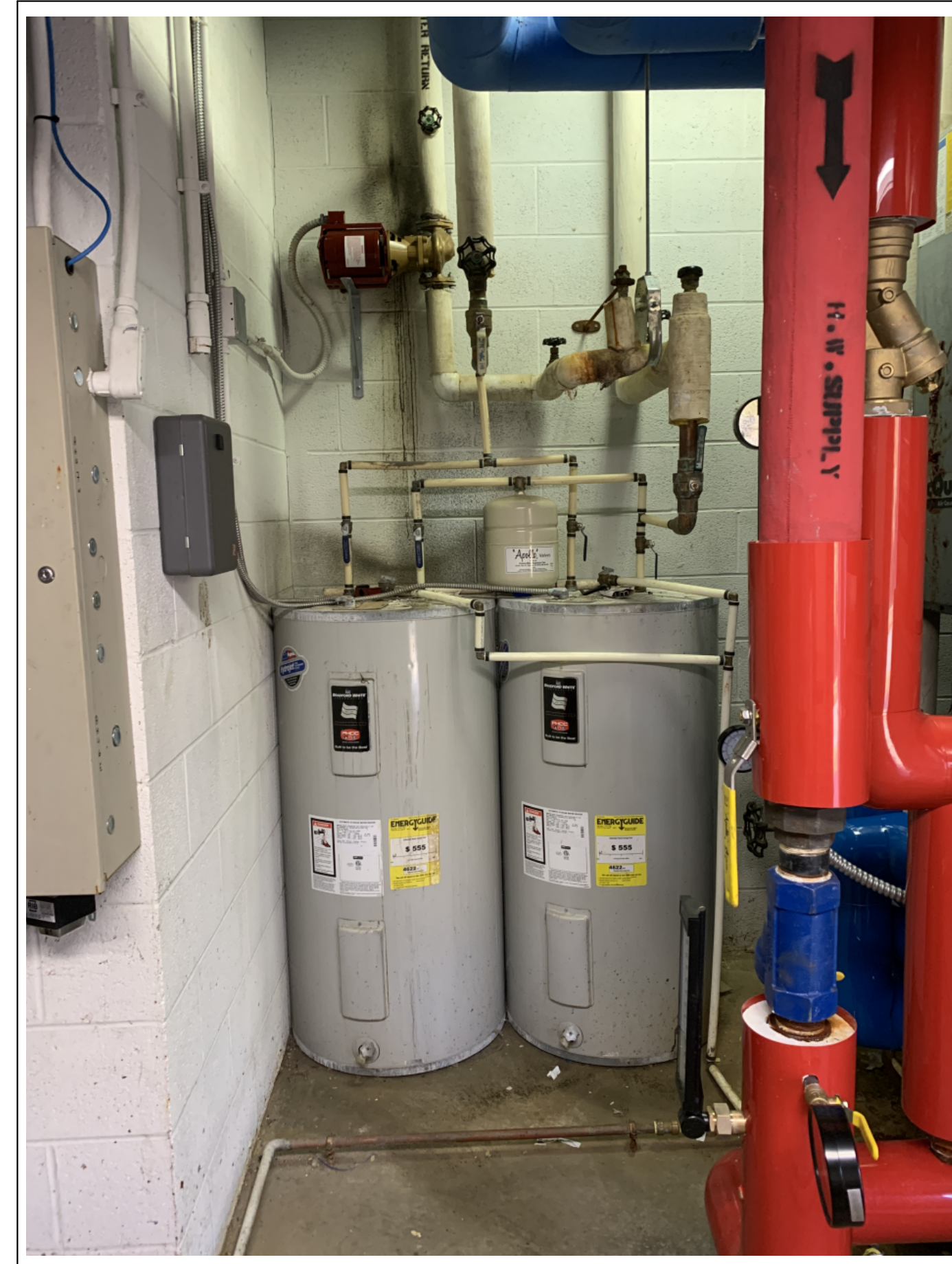
EXISTING ELECTRIC WATER HEATERS
