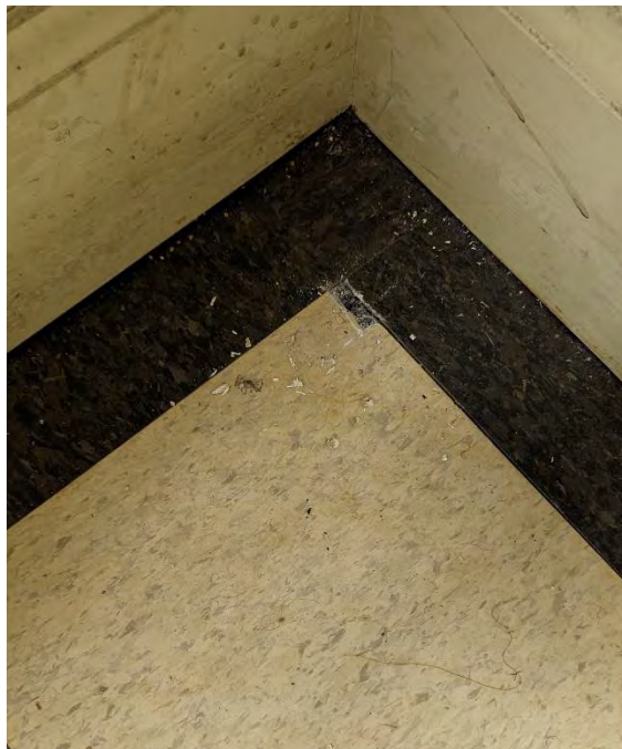
12” Cream Mottled Floor Tile and Asbestos Containing Black Mastic
