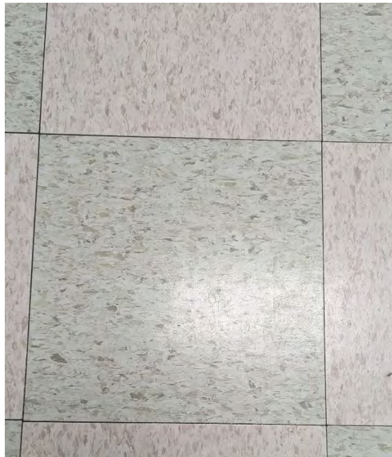
12" Light Green Floor Tile and Asbestos Containing Black Mastic
