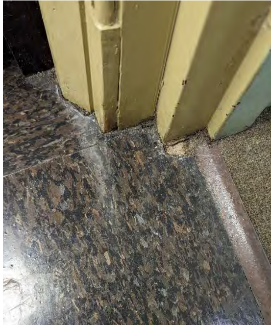
Asbestos Containing 12” Dark Brown Mottled Floor Tile and Black Mastic
