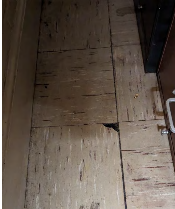
Asbestos Containing 12" Tan W/ Brown Streak Floor Tile and Black Mastic
