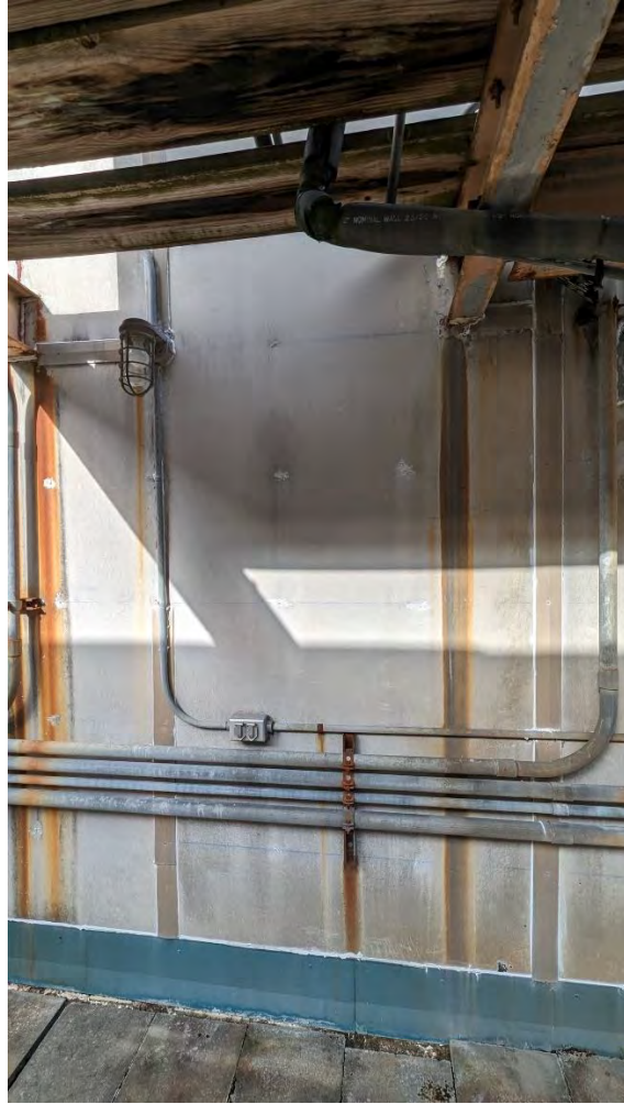
Assumed Asbestos Containing Transite Wall Panels
