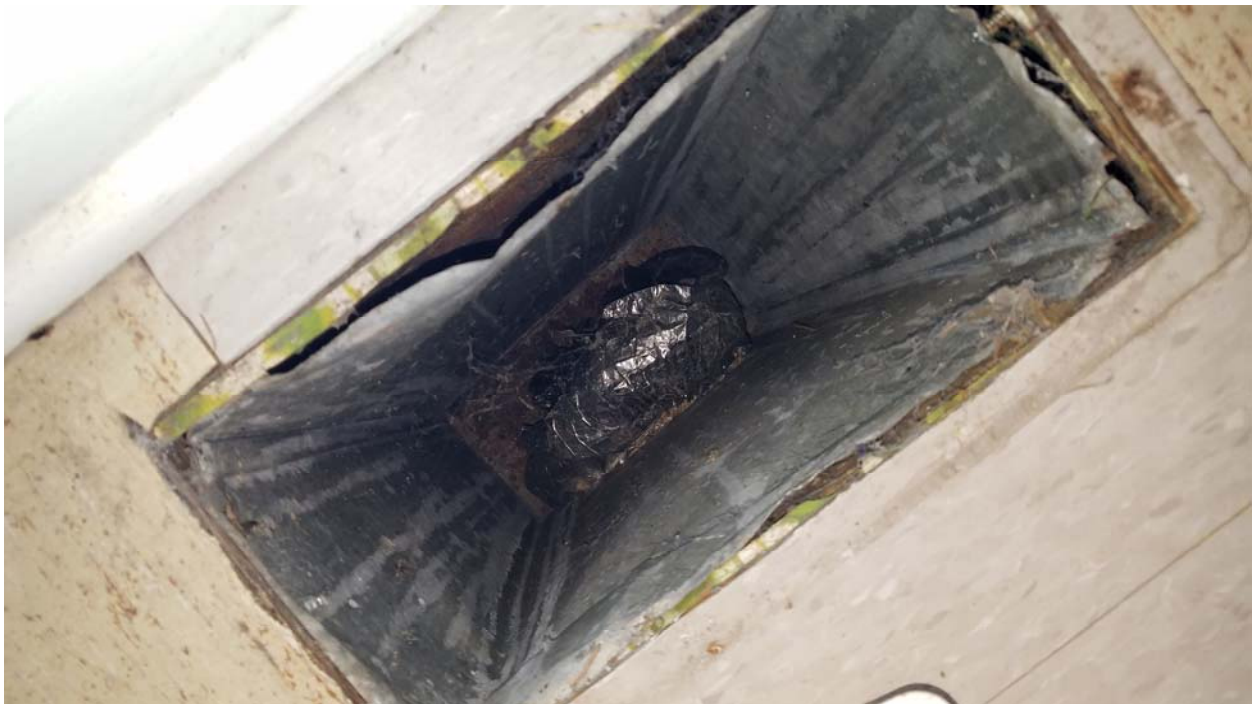
Debris in floor vents.
