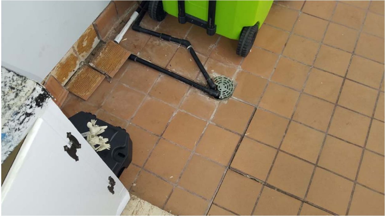
Sagging kitchen floor.
