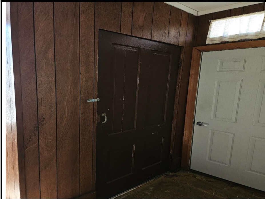
9. Bathroom 3 Brown Side of the Door
