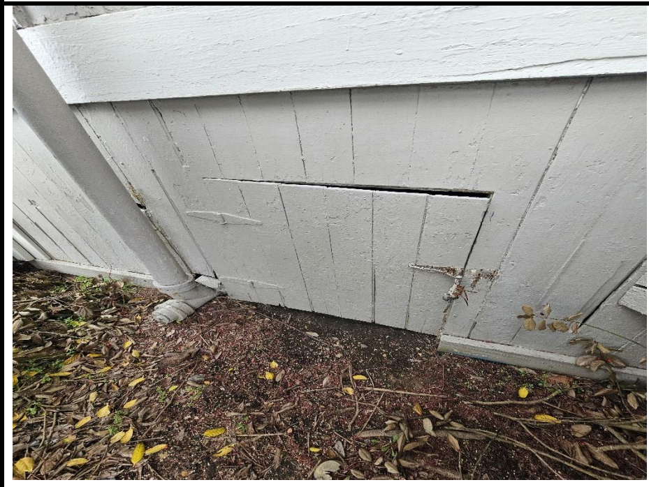
20. White Exterior Crawlspace Access Door
